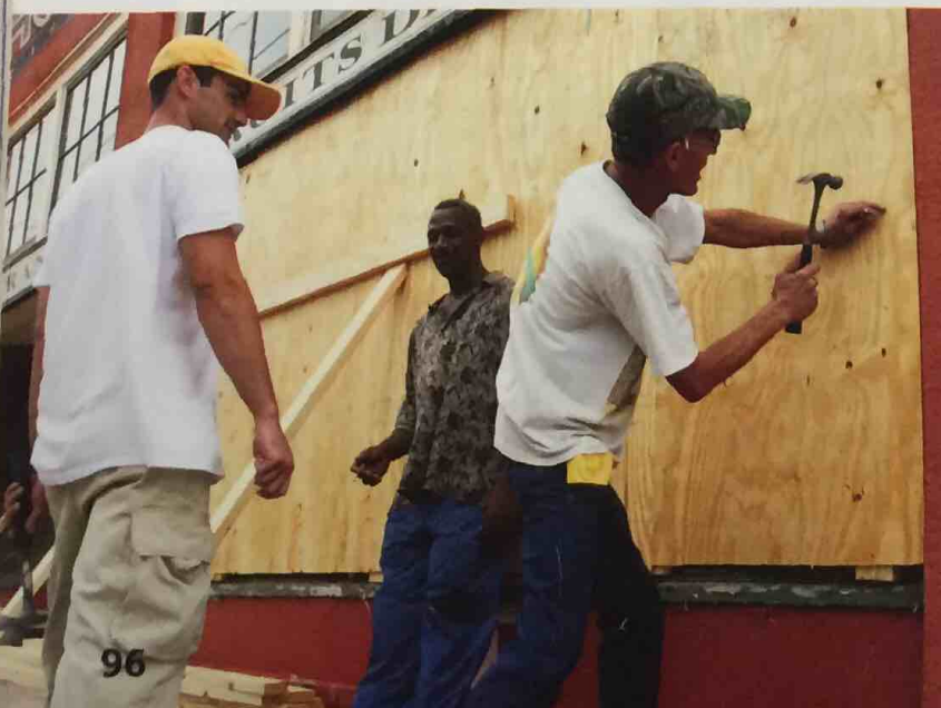
Figure 11 These store owners are boarding up their windows to protect the windows from strong winds during a hurricane.
